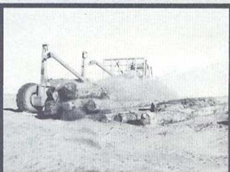
EMPTY — Entire load is safely on the ground a few minutes after Transporter stops. Portable ramps may now be reloaded and another trip begun.
